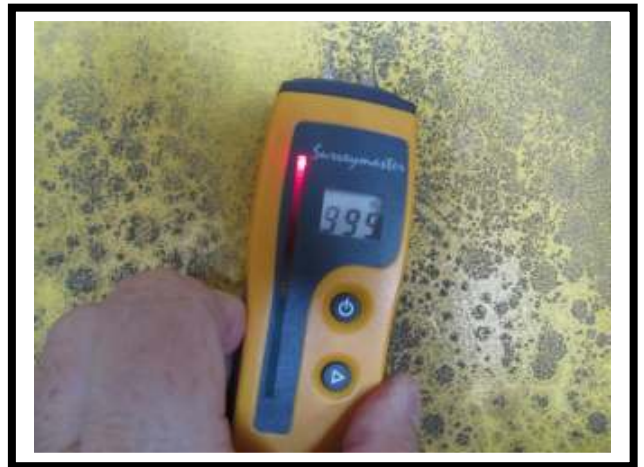
High Moisture Levels 2 Months After Flood
