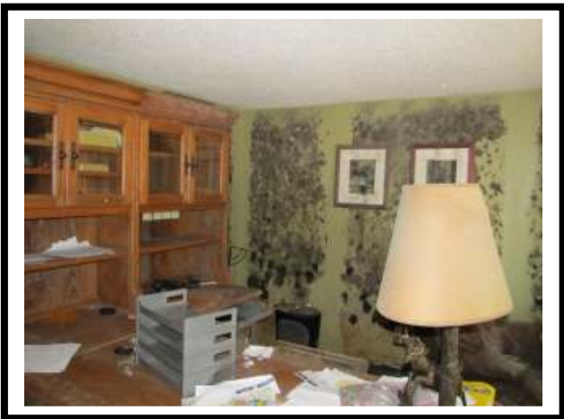
Heavy Mold Contamination On All Walls
