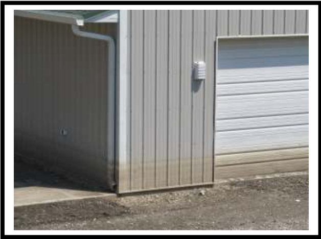
See Water Line On Building Walls
