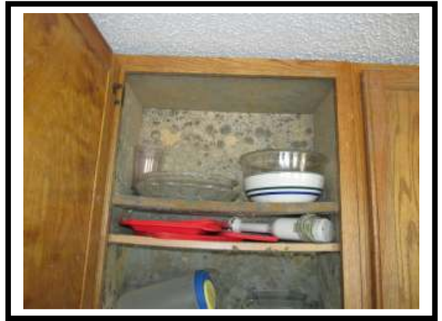
Heavy Mold Inside All Cabinets, Closets, Inc
